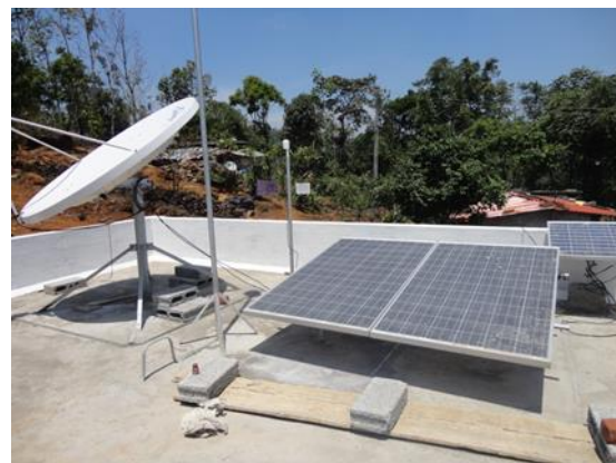
Figure 10-1: Photograph of Satellite communication and solar panel installation in Vallakadavu observatory Kerala
