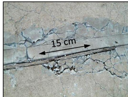
Figure 5-3. D-cracking along a contraction joint in a floor slab.
