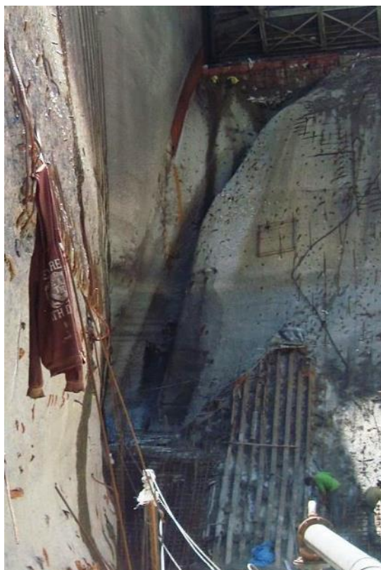
Figure 5-5. Abrasion and cavitation of Gate 1 of Maneri Dam, Uttarakhand, after severe 2013 flooding. Reservoir silted up to the spillway crest elevation allowing boulder-size and quartzite material to flow over spillway.
