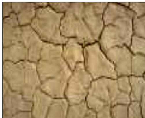
Figure 4-7. Desiccation cracks that form a honeycomb pattern.
