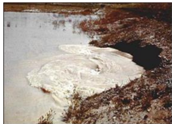
Figure 4-16. Photograph of a whirlpool along the upstream slope of an embankment dam.
