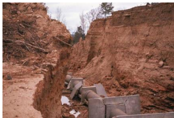
Figure 6-4. Failure of embankment dam resulting from piping erosion along conduit. Compaction around seepage collars is difficult and creates an easy path for water to flow that will initiate backward erosion and carrying of fines. Approximately 25 percent of all embankment dam failures are a result of internal erosion or backward erosion (piping) associated with conduits.
