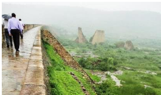
Figure 5-7. During construction (which began in 1916) the dam had a breach in 1917. Causes of the breach noted uplift pressures on a thin clay lens in the sandstone. As a result, methodically placed buttresses were constructed at various chainages along the length of the masonry. (Tigra Dam, MP)
