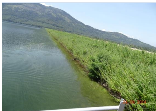
Figure 4-12. Woody vegetation on the embankment is detrimental to the health of the dam by creating seepage paths along the roots and overall impedes dam safety inspections.
