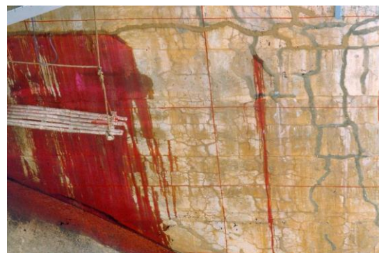
Figure 5-4: Positive identification of ASR at Rihand Dam, India using red dye to demarcate areas of cracks and seepage. no known cure except to minimise exposure to moisture to slow down reaction.
