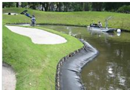
Figure 4-53. An example of use of geo-tubes (filled with dredged material) for bank protection ( http://erosionbarrier.com )
