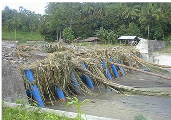
Figure 4-8. A sabo dam which seized debris at the time of floods of 2003, Ormoc, Leyte in Philippines (Courtesy: International Sabo Network website)
