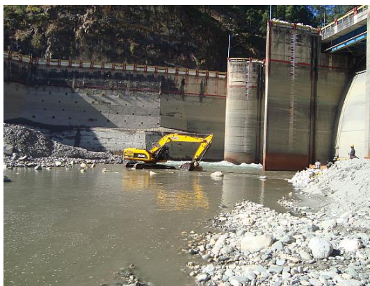
Figure 3-8. Sediment deposition at Maneri Bhali I after the flood. Upper picture shows deposition of fine sediment over coarse sediment layer, while lower picture shows deposition of coarse sediment and boulders near the dam area reaching up to the spillway crest
