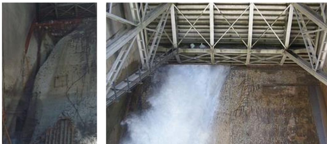
Figure 4-63. Abrasion of spillway glacis (left picture) and malfunctioning of gates (right picture) in Maneri Bhali Stage I (India)
