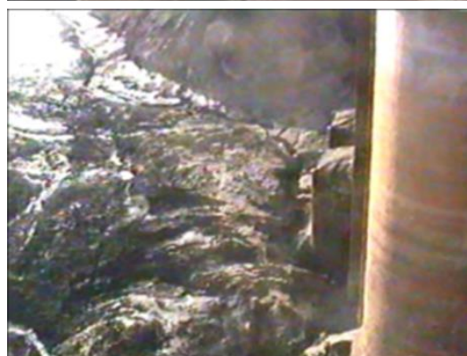
Figure 6-16. Deposition in front of power intake and scour sluices (in 1991)
