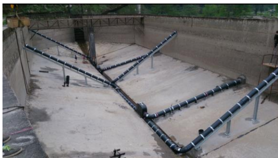
Figure 4-66. Sluicers, installed in the desilting basin (Courtesy: SediCon)
