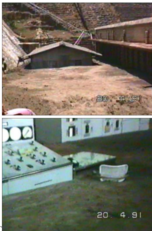
Figure 6-17. Sediments, deposited in and around powerhouse premises as a result of hazards during the flushing
