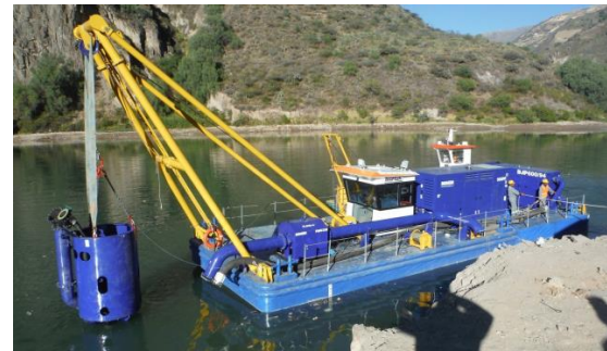
Figure 4-33. A modular dredger with pump in the Tablachaca dam in Peru ( https://youtu.be/UlqvF0Xq_QM )
