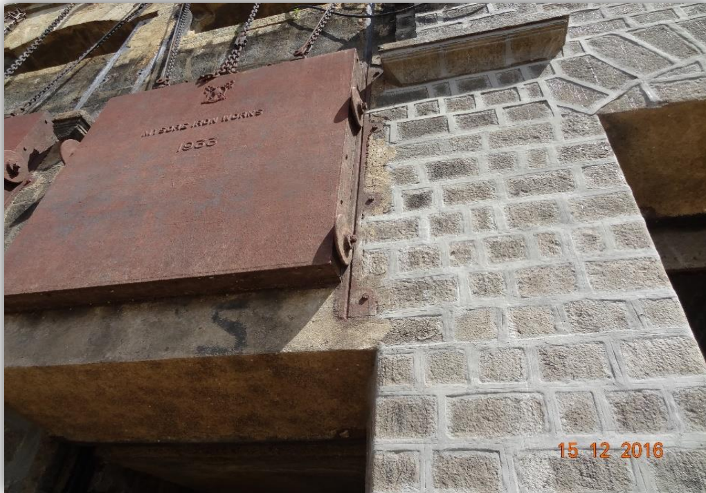
Existing +114' gates presently welded in position. The wheels and the grooved wheel tracks on the right side are visible. Similar track exists on left side also.
