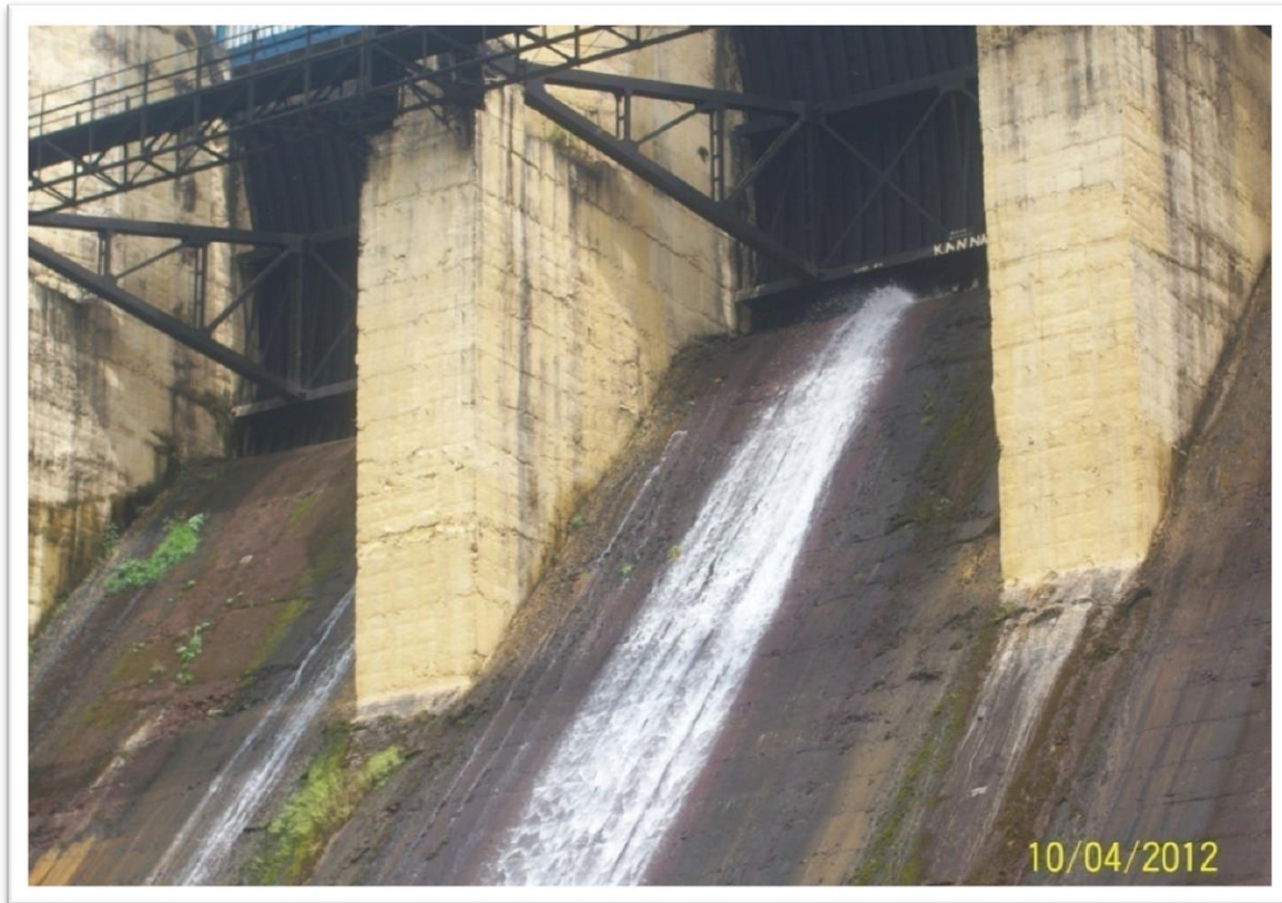
Figure 17 – Photograph showing damaged rubber seal of spillway radial gate
