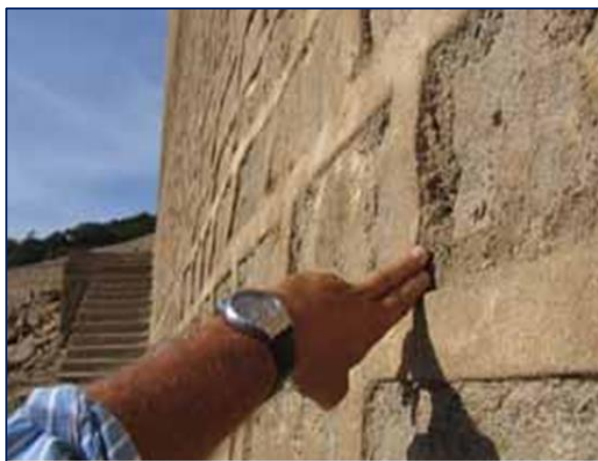
Figure: 1- The stone masonry blocks at the upstream face before being covered by Geo-membrane.
