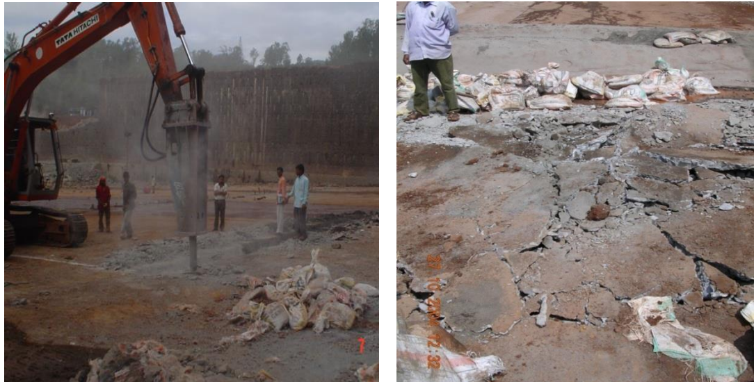
Figure 12: Breaking of reinforcement to enable concrete excavation and Face opening for concrete excavation is done
