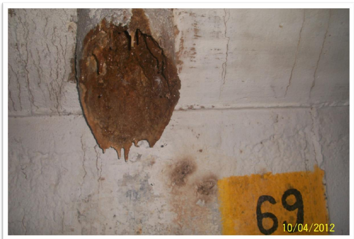
Figure 14 – Photograph showing choked porous holes
