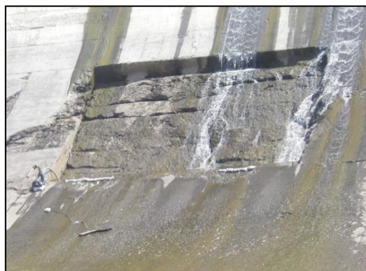
Damages observed in dewatering bay No. 5
