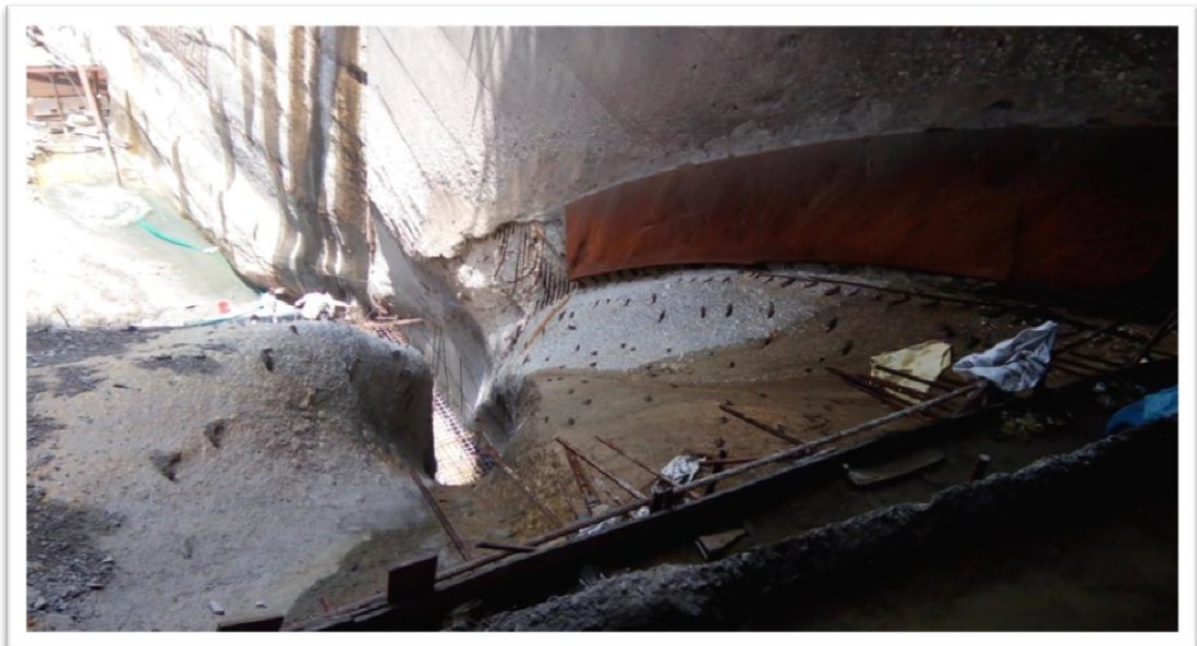
Photograph 1 shows the damages in Spillway bay no-1
