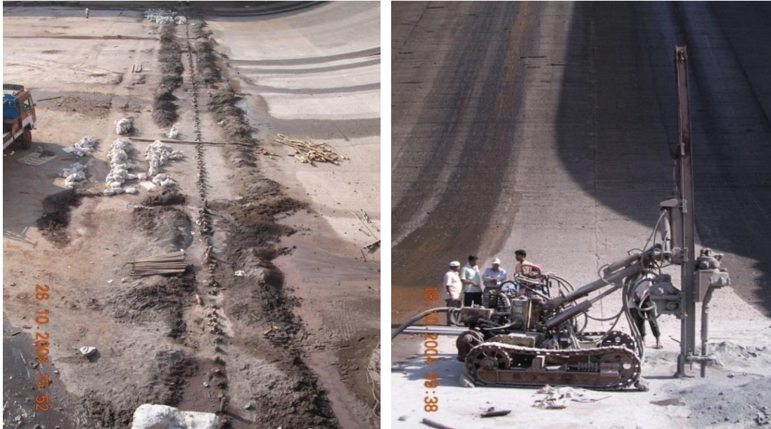
Line Drilling 115 mm dia 400 mm c/c upto full depth to provide separator between Dam & excavation plot
