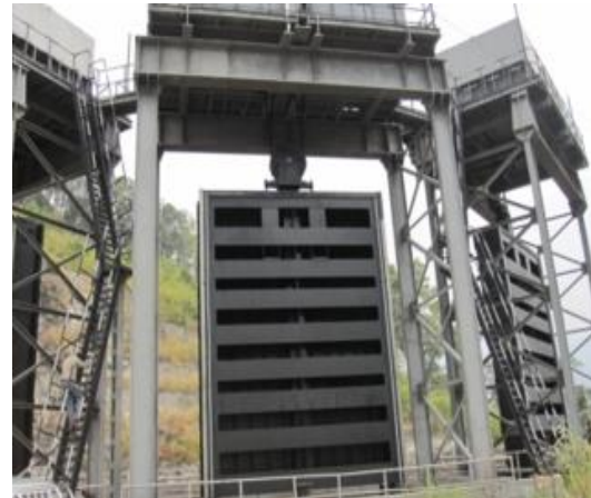
Figure 7-2: Vertical Lift Gate
