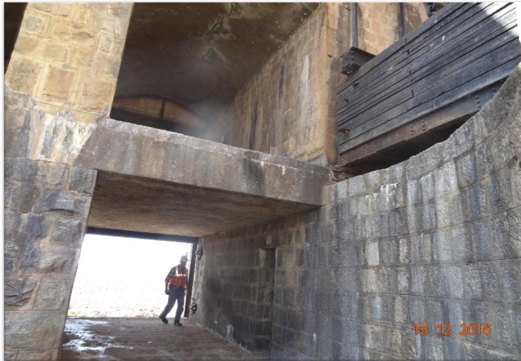
+103' & +114' sluices openings looking from d/s side. The counter weight is visible in suspended condition next to +114' sluice (to be removed, as it may not allow proper aeration of water nappe discharging from +114' gates.)
