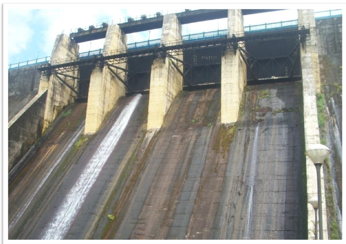
Figure 10 – Photograph showing dam body seepage at spillway portion
