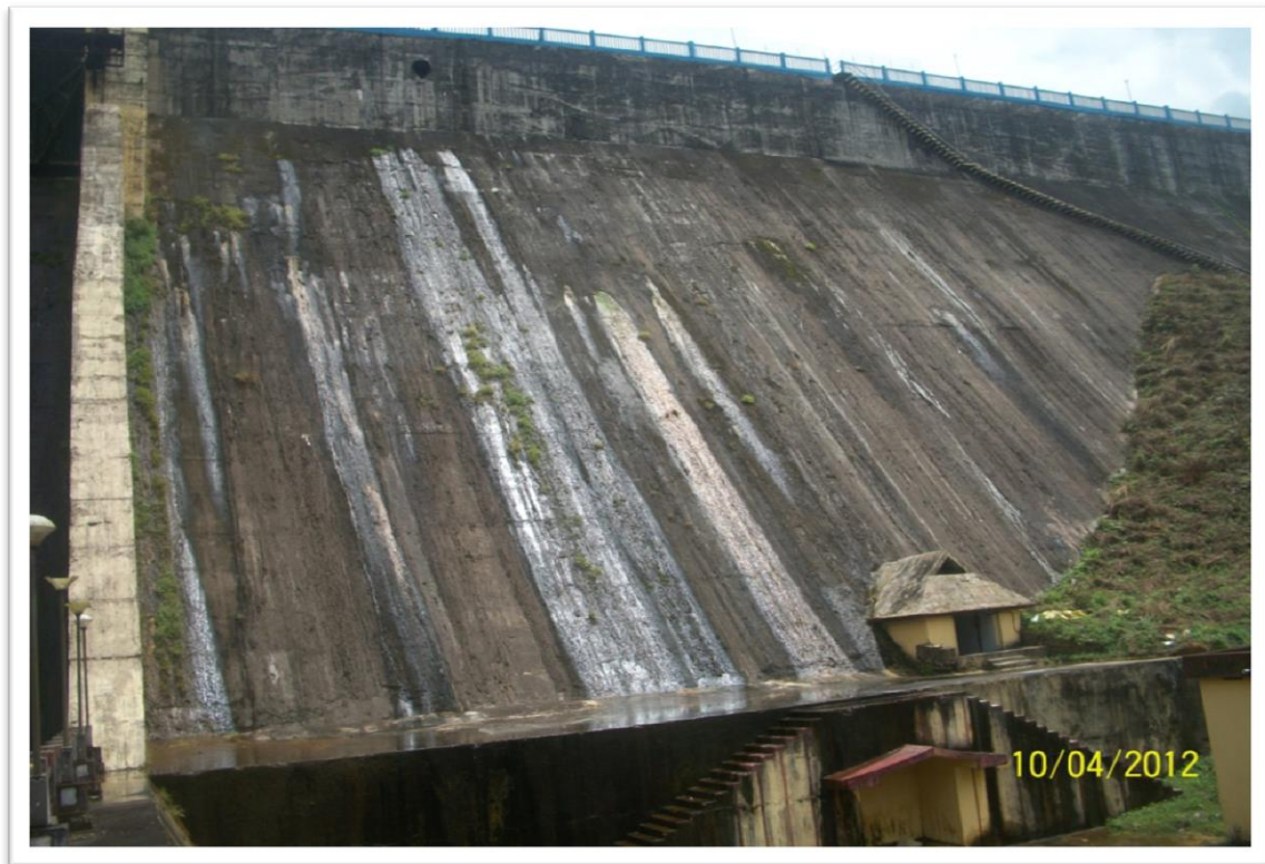
Figure 9 - Photograph showing dam body seepage behind a NOF block
