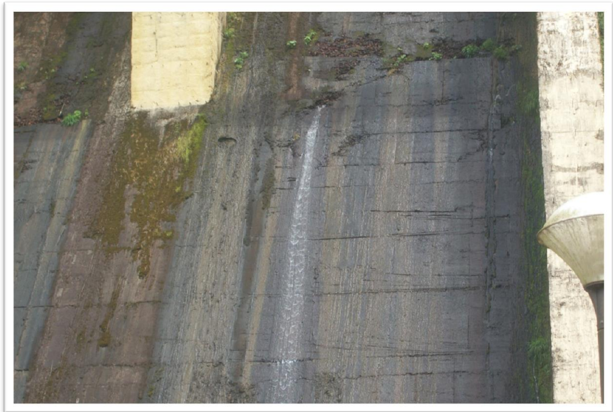
Figure 15 – Photograph showing deteriorated glacial on spillway portion
