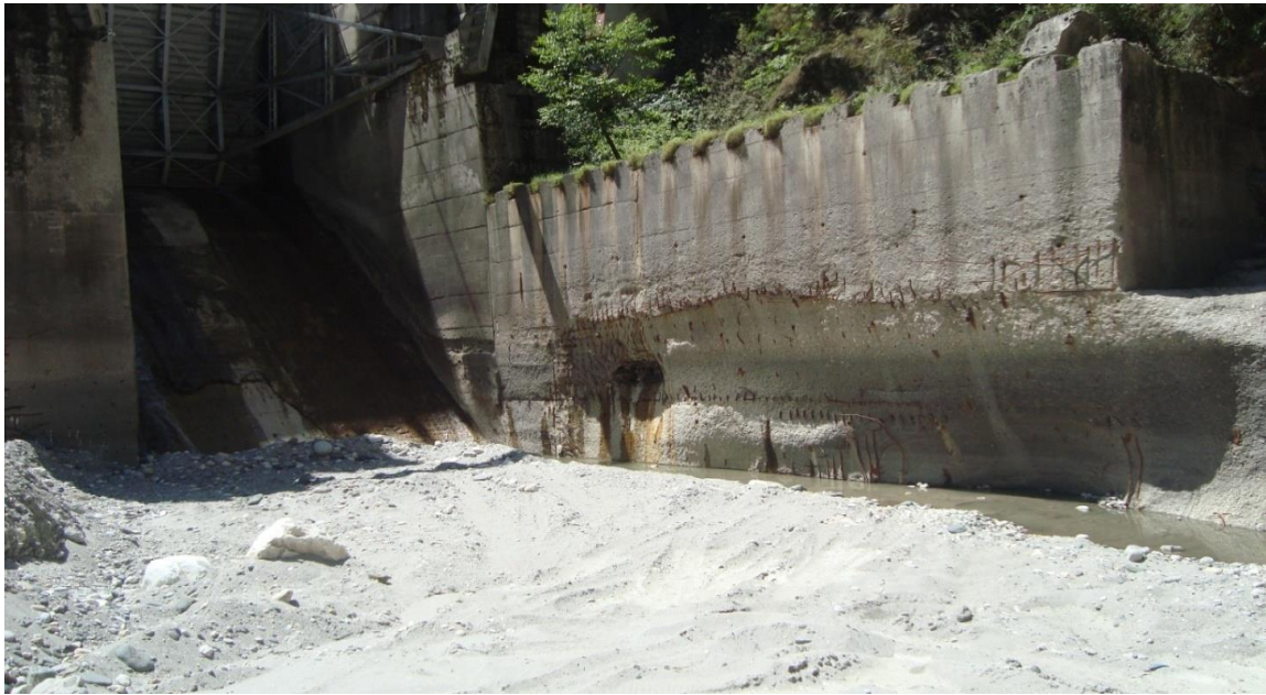
Photograph 5 (Damaged Training wall)
