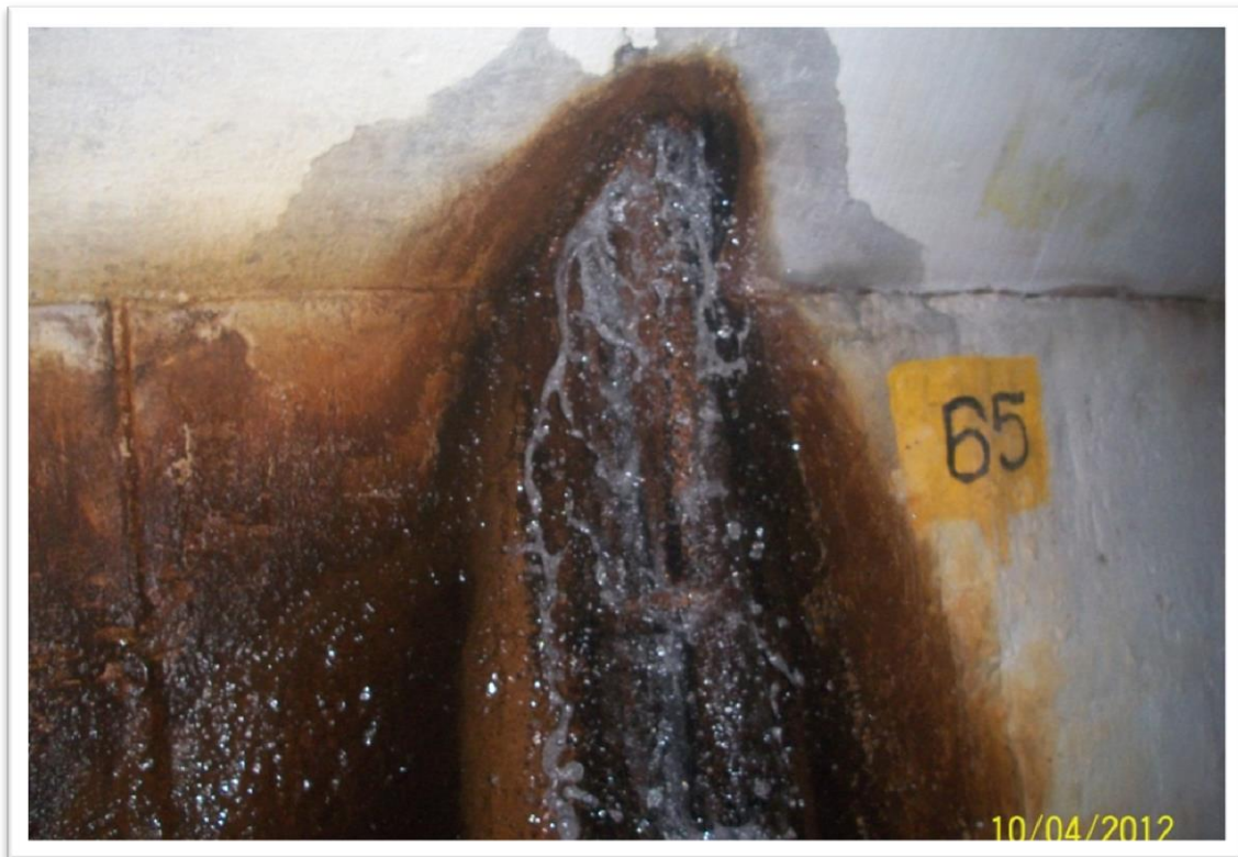
Figure 11 – Photograph showing excess seepage through the gallery drainage holes
