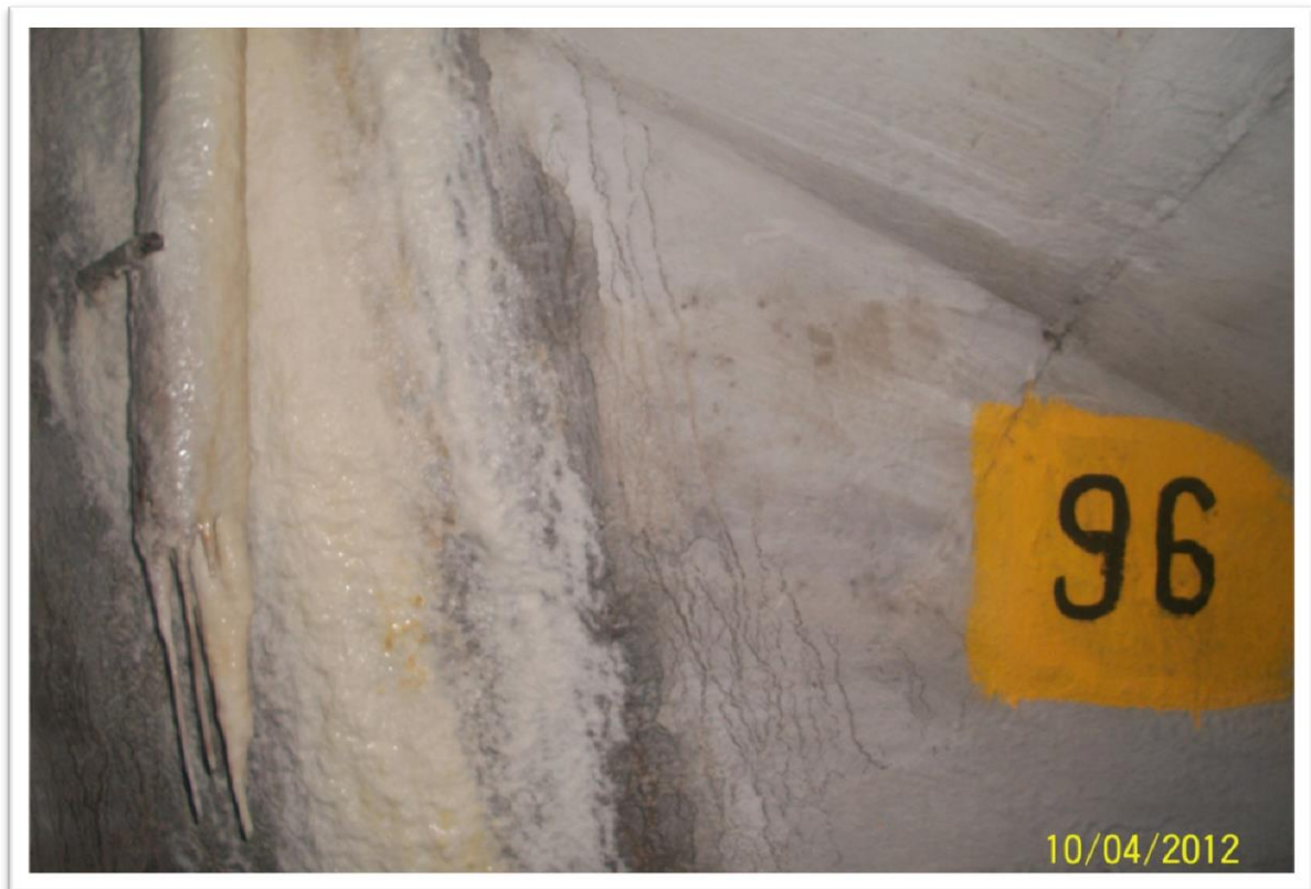
Figure 13 – Photograph showing choked porous holes
