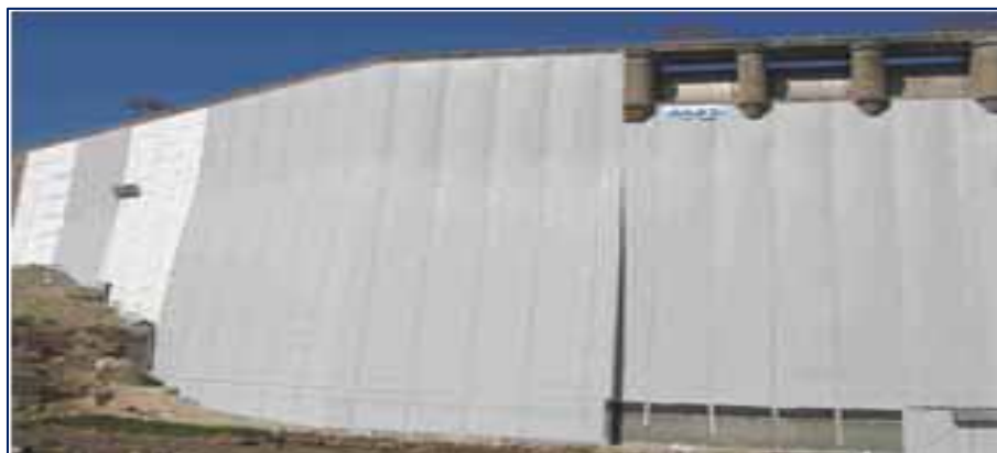
Figure: 3- The waterproofing PVC Geo-composite is installed over the Geotextile and fastened with the second component of the patented vertical anchorage system.
