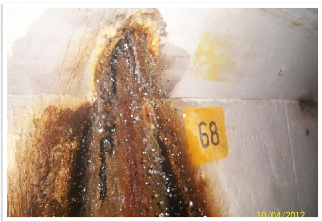
Figure 12 – Photograph showing excess seepage through the gallery drainage holes
