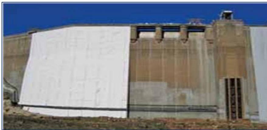
Figure: 2- The vertical anchorage profiles are installed on the u/s masonry dam face of Kadamparai dam at 5.7 m c/c. The anti-puncture geotextile is placed on the dam face between the profiles.
