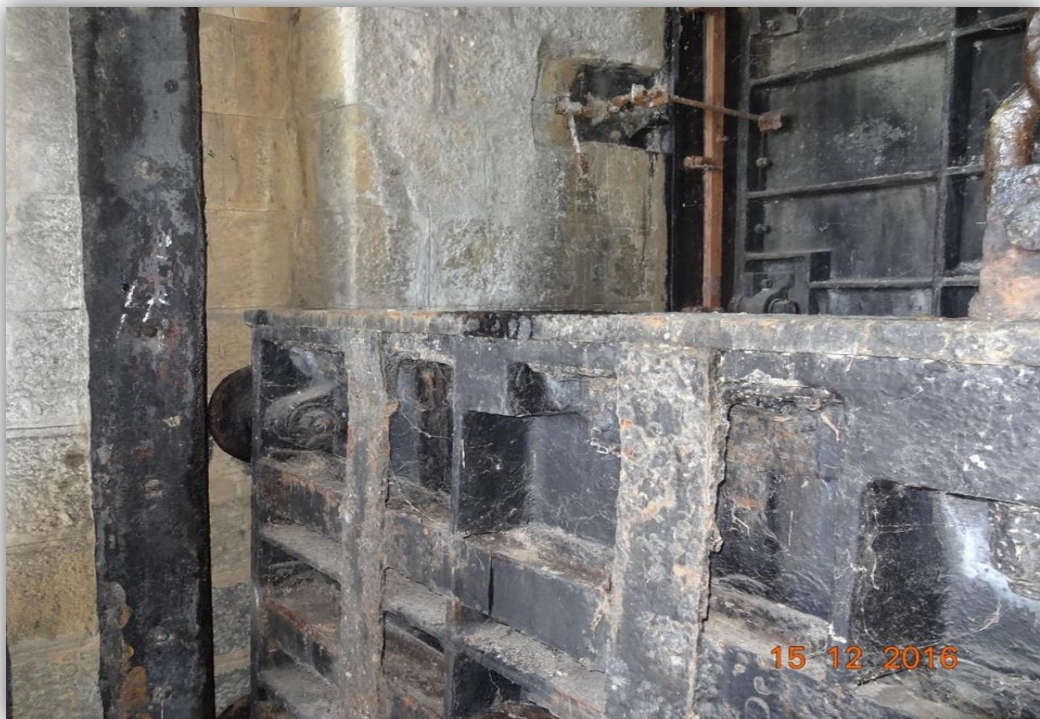
+103' sluice gates in partial open condition with +114' gate in the background - looking from d/s side.
