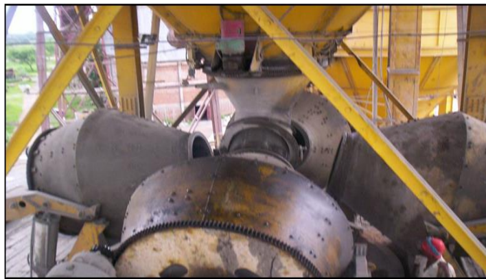
Photo 6: Tilting mixer's in batching plant
