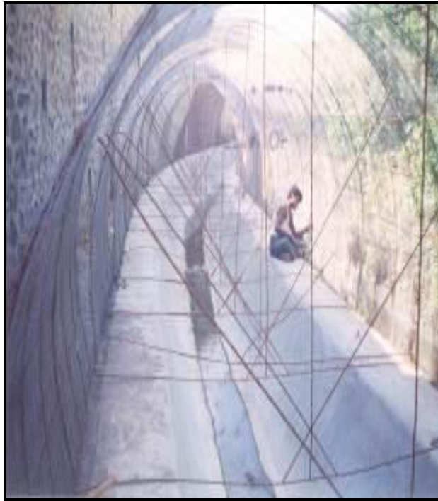
Fig 7.39 Canal or nalla closing by huge ferrocement pipe cast in Situ near Pune
