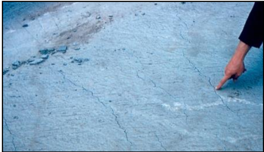
Photograph 4.4.1 C: Plastic Shrinkage crack
